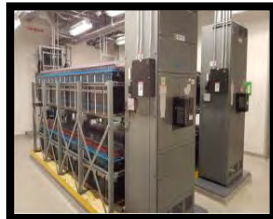
Backup/ Distributed Generation
