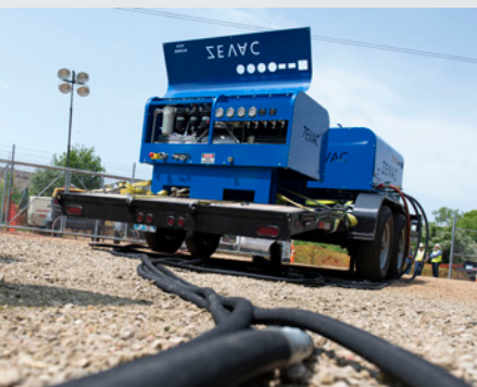
Using innovative ZEVAC vacuum pump technology to avoid gas venting when pipelines are taken in and out of service
