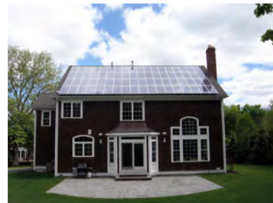
Roof-mounted solar array for large power capacity.
