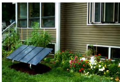
Ground-mounted solar array allows optimal tilt and avoids placement of panels over roofing.
