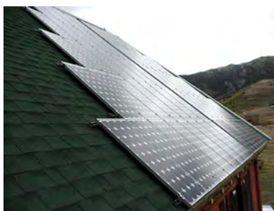
Monocrystalline solar panels.
