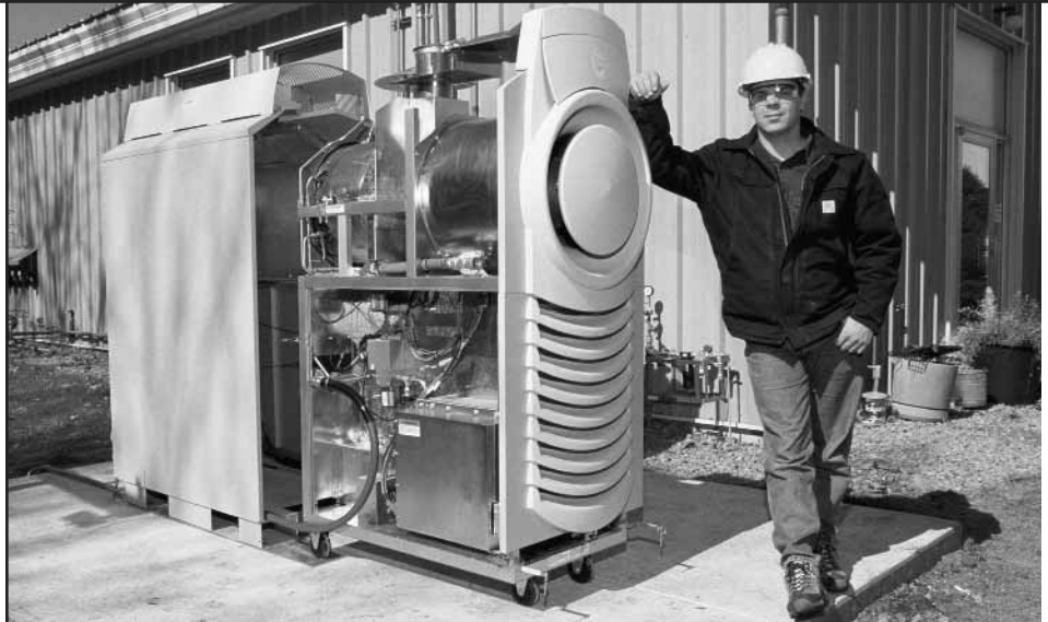
On-site power generation reduces waste.
